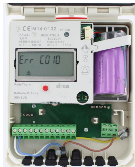
Figure 10: connected flow sensor PolluFlow with voltage supply
